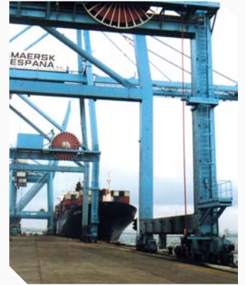
Cable reel with wound rotor torque motor drive in container crane, travel length 327 mts., height 17 mts. Tensión 20 KV.
