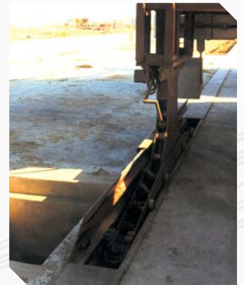
Detail of channel cable with steel cover and lifting device system. Cable voltage 10 KV.
